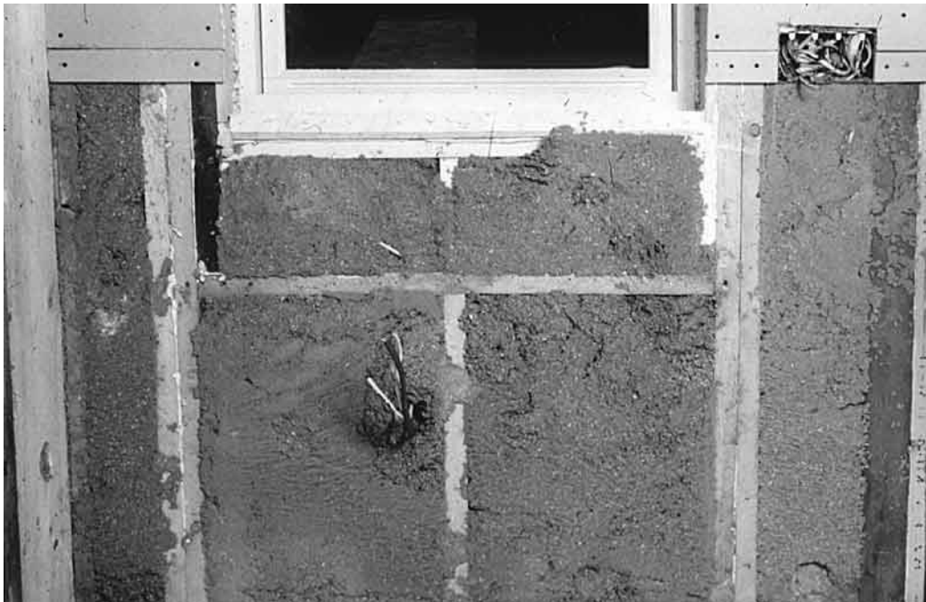
Figure 8: This demonstration wall was blown full of cellulose and then the interior sheathing was removed to inspect the result.
