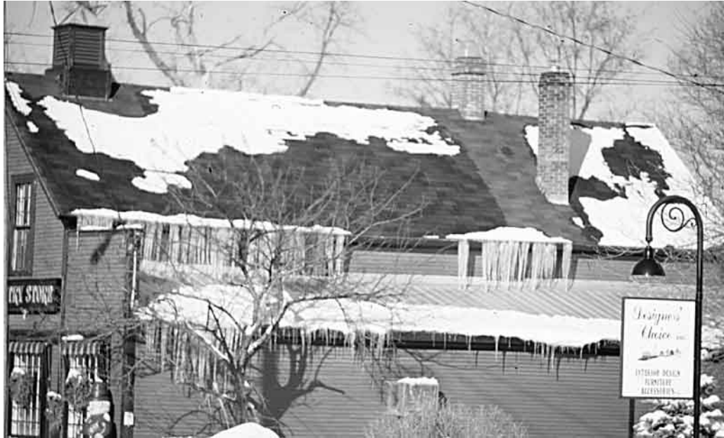
Figure 2: When the snow on a roof melts much more quickly than on those of surrounding buildings, it is evidence of large amounts of heat loss.
