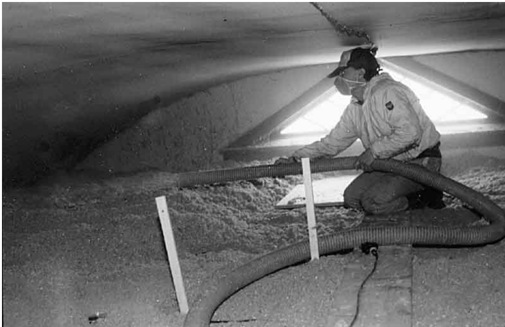
Figure 9: Blowing an attic crawl space. Cellulose does not have to be sandwiched between two surfaces as in a wall or under a attic floor.
