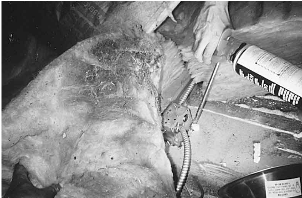
Figure 3: The dirty, stained fiberglass around this electrical fixture indicates that a large volume of air is moving past this spot. The fiberglass acts as a filter, trapping the dirt, much as fiberglass furnace filters do.
