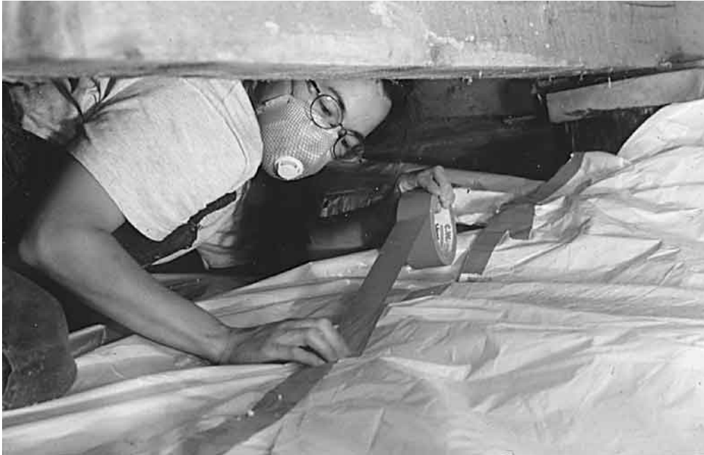
Figure 5: Laying Tu-Tuf, a cross-linked polyethylene sheeting, in a crawl space. Tyvek tape works well for taping edges together.
