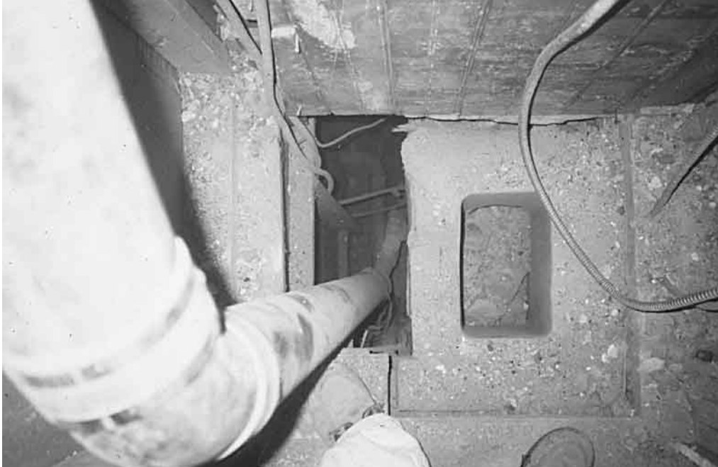
Figure 6: Plumbing chases can be large, problematic holes in the thermal envelope.
